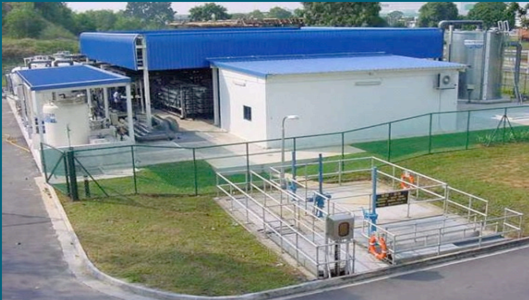
Demonstration Plant, May 2000
